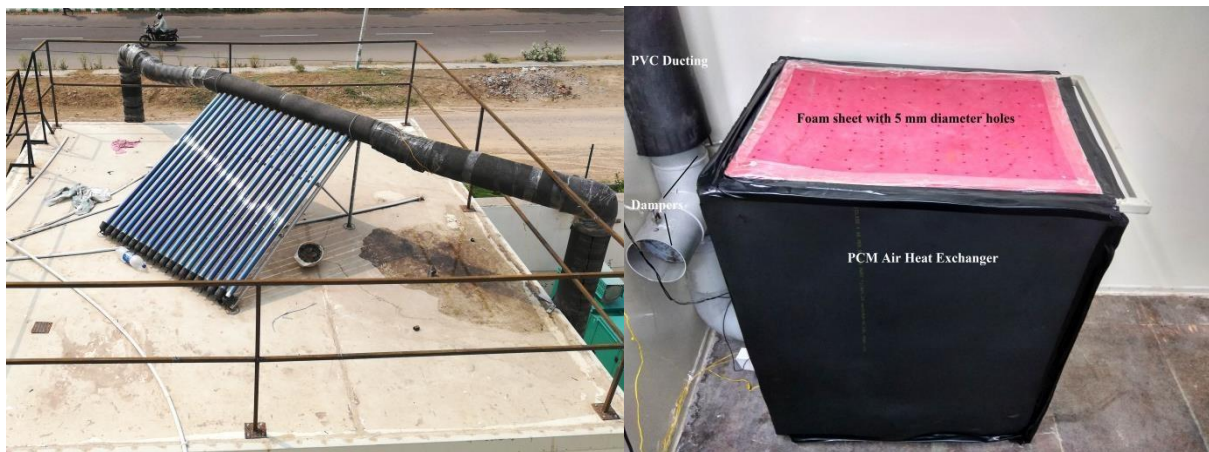
Figure 3: (L) ETC solar collector system with ducting (R) PCM air HX with Nitrile rubber foam insulation and dampers to switch the air circulation during night-time.
