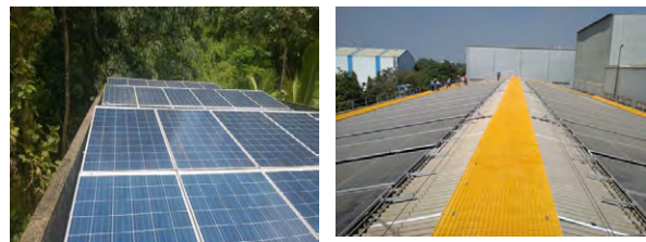
Figure 3: Power plant with (a) No access to far end PV arrays, (b) proper walkways for accessing PV arrays
