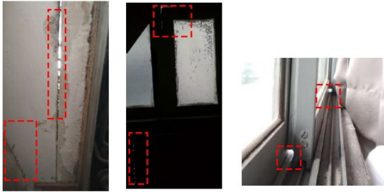
Figure 8 Leakage pathways through window perimeter
