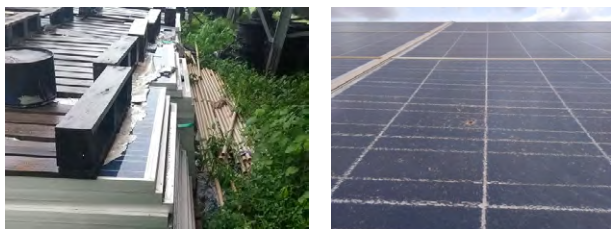
Figure 8: Faulty PV panels in a 6 year old utility scale power plant
