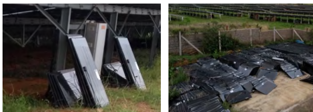
Figure 7: Faulty PV panels in 7 years old utility scale power plant
