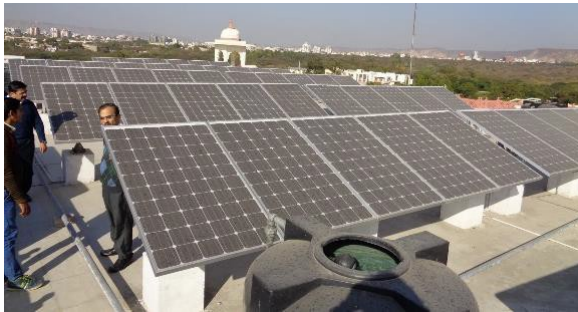
Figure 9: SPV system at the rooftop
