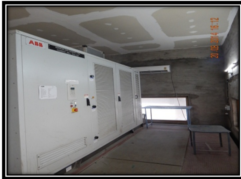
Figure 5: VVVF (MV) DRIVE
